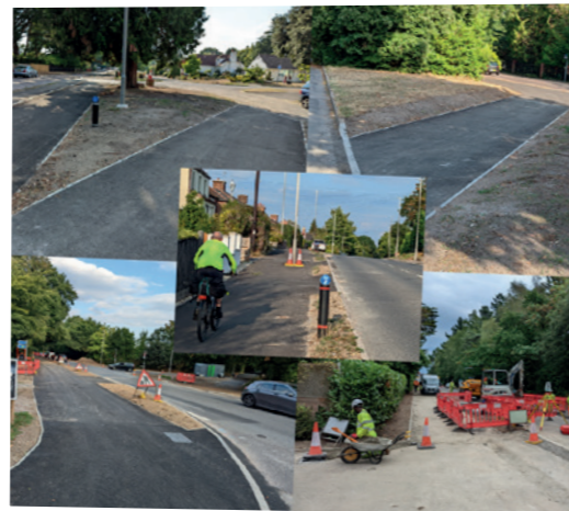
The new cycling and walking route under construction on Wimborne Road, Ferndown.
