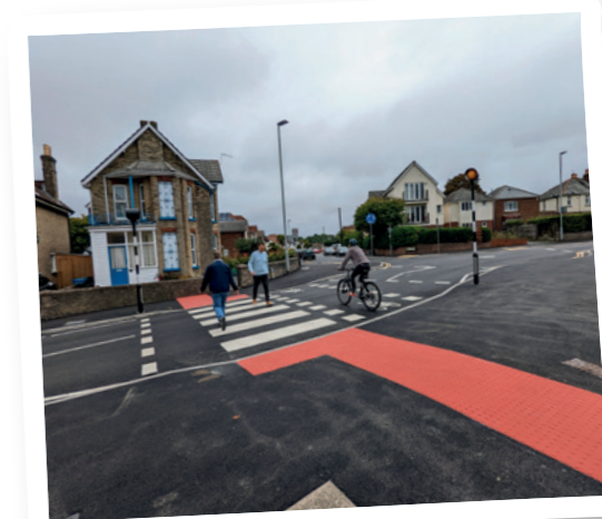
The new parallel crossing on St Mary's Road near the Garland Road junction.
